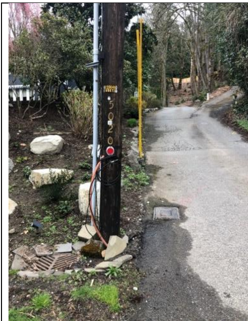
Photo 7. View of private access driveway on north end of Project Site where the piped watercourse is located as evidenced by the two drains. Looking east. Photo taken 3-17-22.
